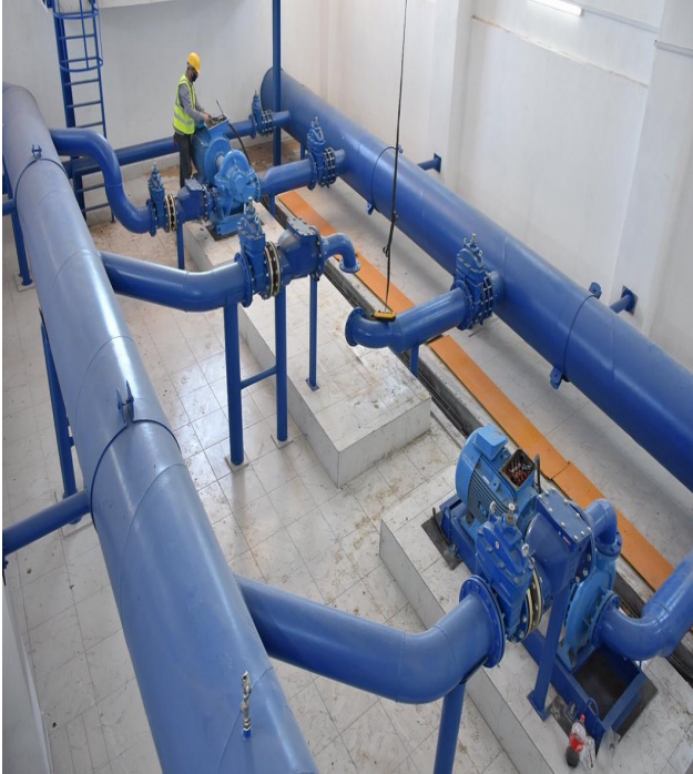
Terfi Merkezi Pumping Station
